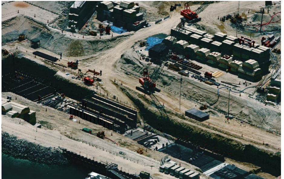
JBR District Cooling Piping Culvert (under the Marina Channel)
