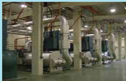
Jumeirah Beach Residence - District Cooling System
