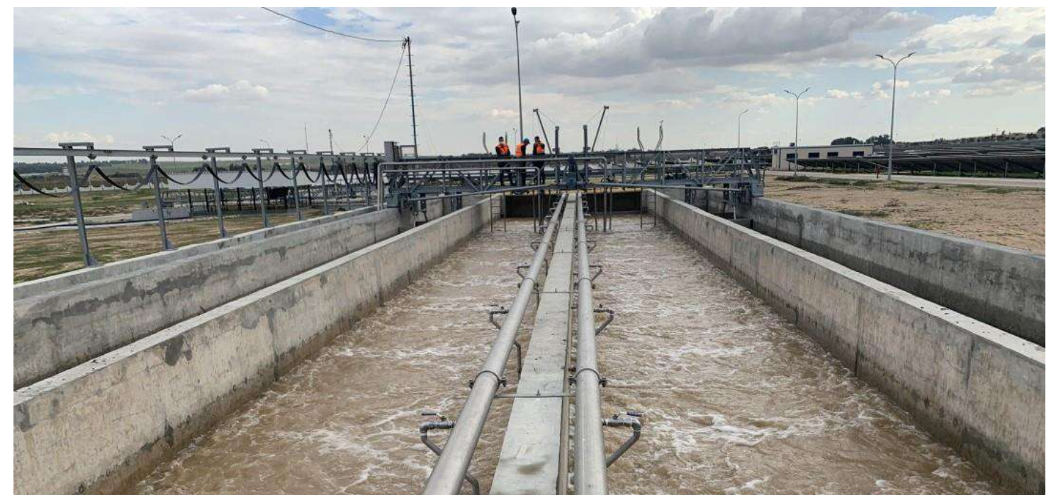
Commissioning of the plant in December 2020
