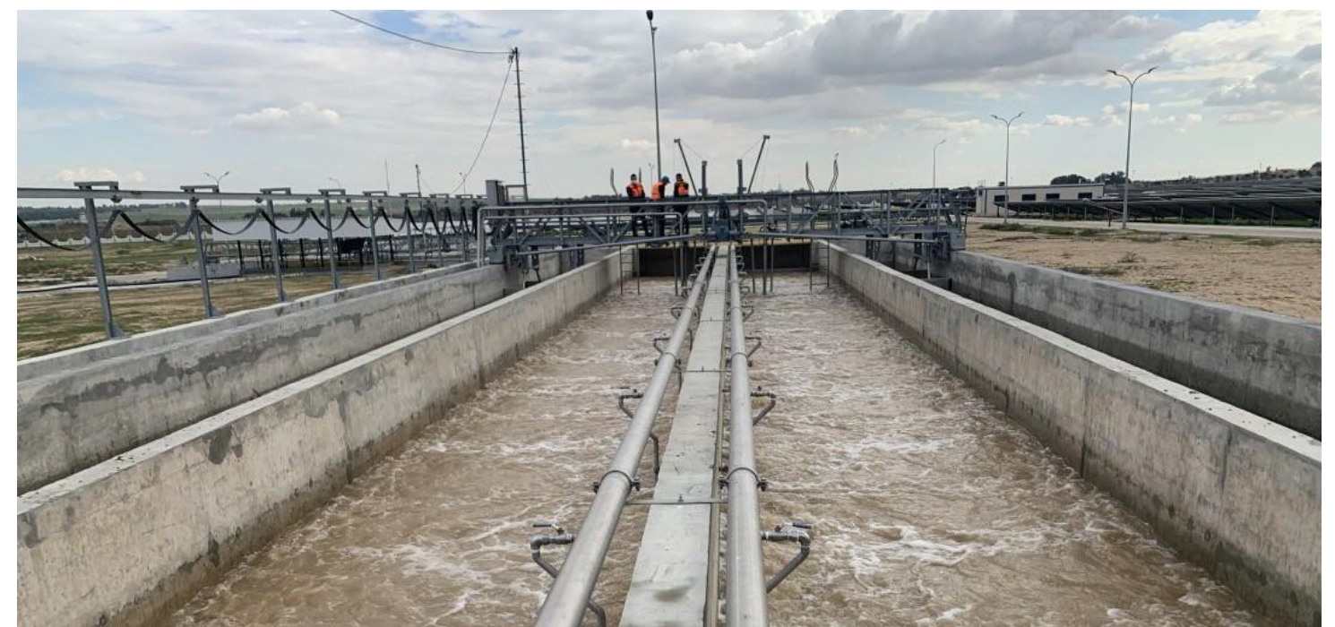
Commissioning of the plant in December 2020
